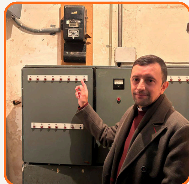
Excolegiata Parish of Santa María la Mayor, Alcañiz – Donation of €6,000 from the SAMCA Foundation for the replacement of the electrical switchboard
